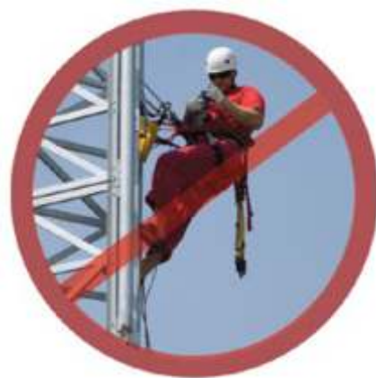
The Viavi Solutions RFoFiber reduces risky cell tower climbs letting technicians test safely from the ground
